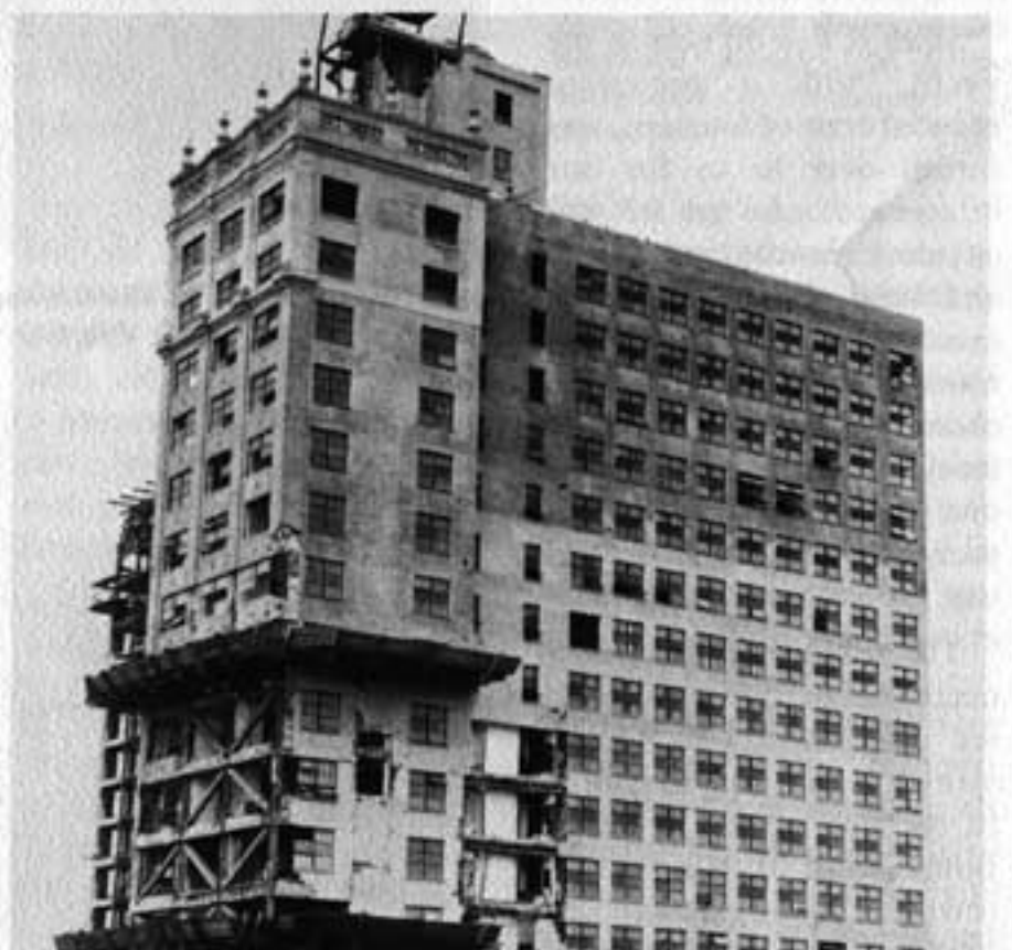
Hit broadside by the wind, the upper stories of the 17-floor Meyer-Kiser building buckled and later had to be torn off. Scaffolding prevented rubble from falling on pedestrians. (All photos: Romer Collection, Miami-Dade Public Library.)
