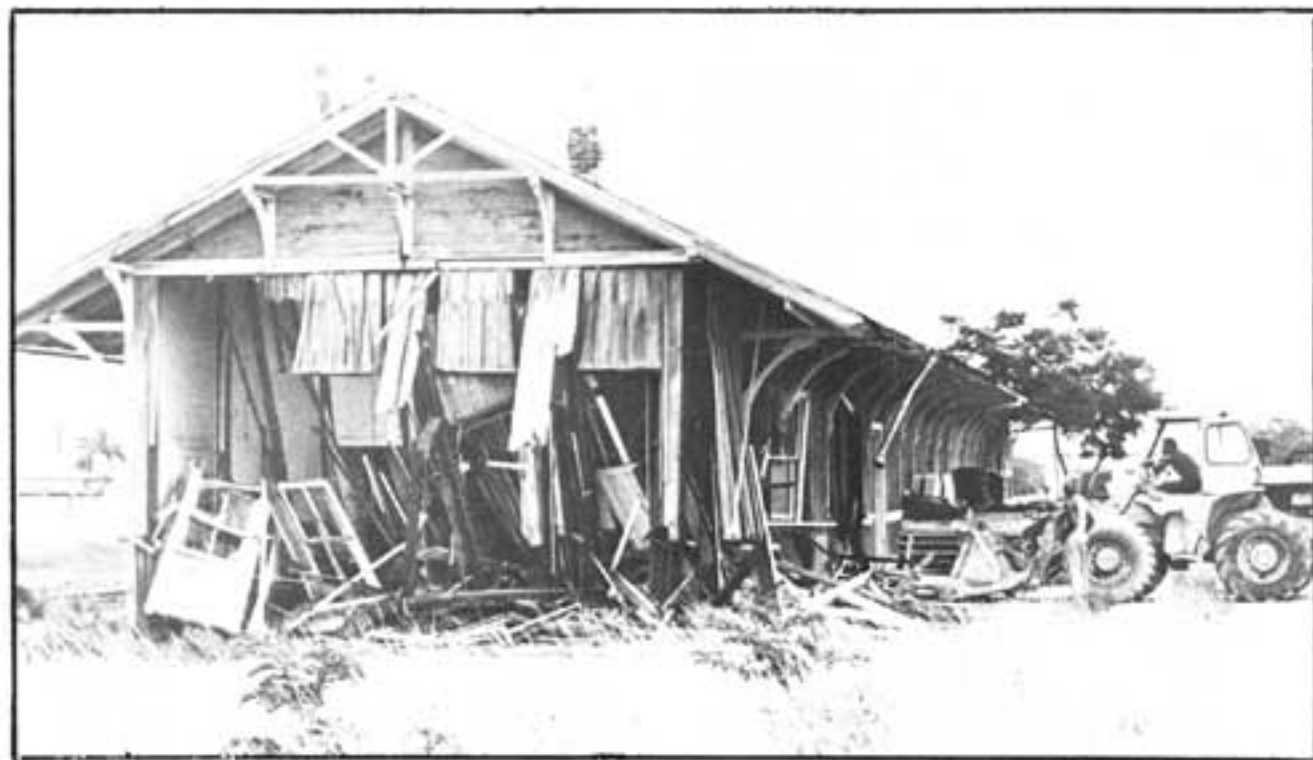
On June 23, 1976, a front end loader began the demolition of the old Florida East Coast Railway station. When the demolition began, the office furniture and records were still inside and a full tank was hooked up. Area residents had the night before appeared before the Homestead Council and been granted their endorsement of the effort to preserve the depot. (Photo courtesy of The Homestead News Leader.)
