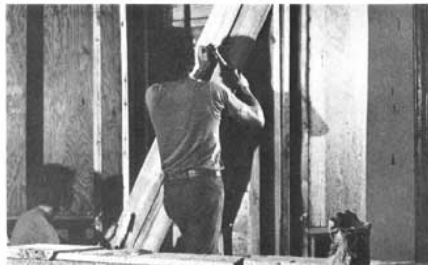
With shop set up in the gallery proper, James Tobak and Tom Slingerland begin construction of the display cases for the period. Wood siding varies horizontally, vertically and on the diagonals depending on the period of South Florida history being explored. To the left are displays from the original gallery.
