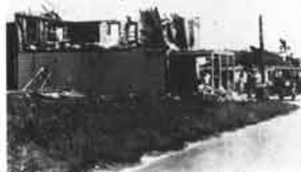
Leon Mock family lived above their store in Goulds. After '26 blow they converted it to one-story house.
