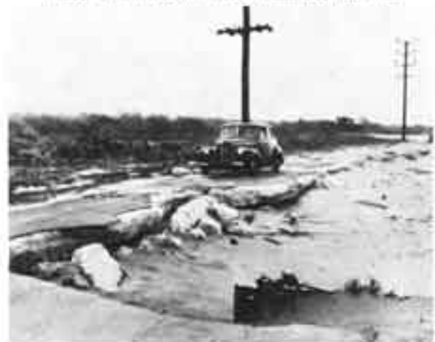
Highway above Baker's Haulover was washed out in 9-17-47 storm.
