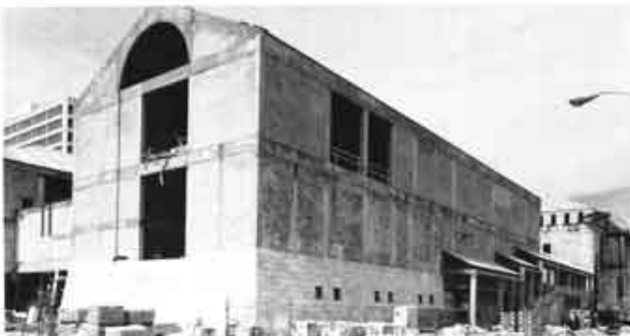
On August 15, 1981 this is how HASF's new museum looked. You are facing southwest and can see the art center on the left and the wall bordering the elevated piazza which is the entrance level for the three buildings. The north end of the library shows on the right.
