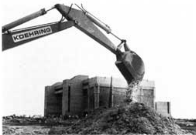
Earthmover is already busy leveling ground for the second building, Deuxieme Maison, while work goes on at Primera Casa. PC, as the building is called, housed all functions of the university at first. Classrooms, student union, library-auditorium and two lab buildings came later.
