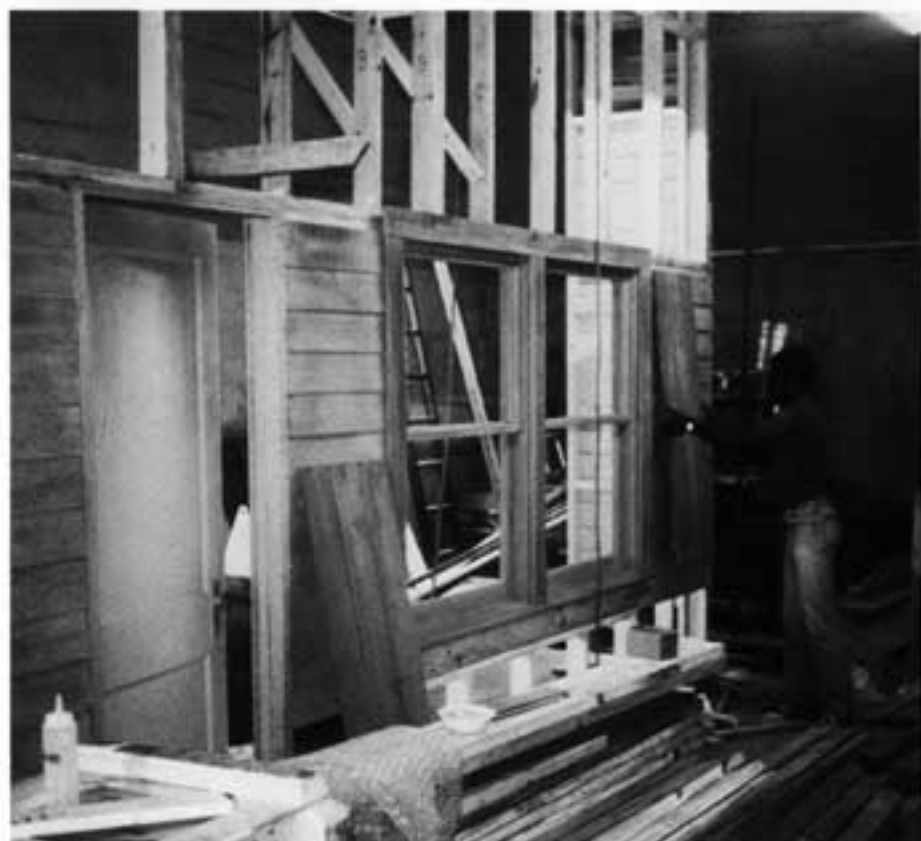
Each board, stud, window sill, door frame was numbered and dismantled for easy re-assembly. The fabricators, Presentations South, Inc., are the only museum producers in the south.
